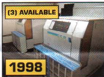
Ingersoll-Rand 30 HP Rotary Screw Air Compressors
