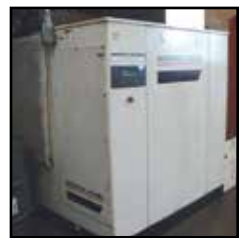
Ingersoll Rand SSR-EP75 Rotary Screw Type Air Compressor
