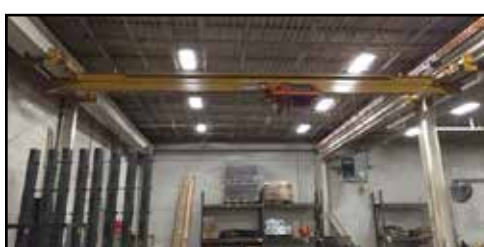
3-Ton Overhead Bridge Crane
